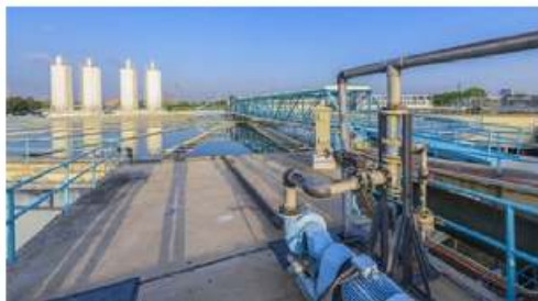
Utilities (Power, Telecom, Gas, Water)
